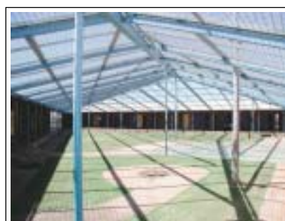
Sky bars over Unit One. The construction of a fortified perimeter fence made the sky bars superfluous to security needs.
