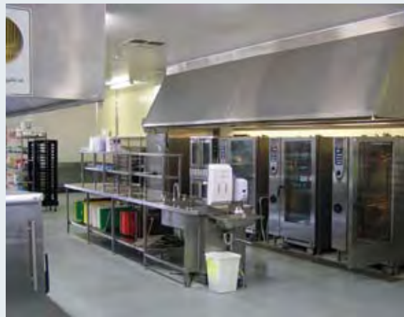
Maintenance issues were identified in the kitchen, including inoperable ovens.
