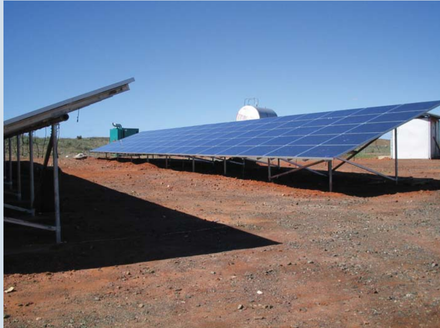
Solar panels at the Mt Morgan work camp – a major initiative to minimise the camp’s environmental impact.
