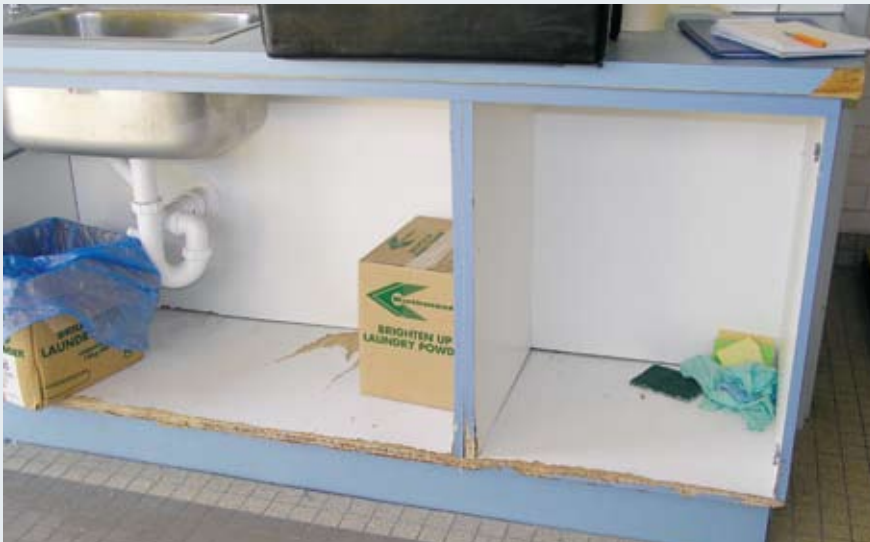
However, many other areas of the centre were in urgent need of maintenance or upgrade. Shown here are laundry cupboards in self care accommodation.
