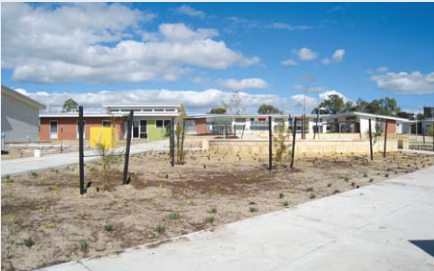
A view from inside the new pre-release unit close to completion. The physical design of the unit resembles a community living environment similar to that seen at Boronia Pre-release Centre for Women [4.16] – [4.17].
