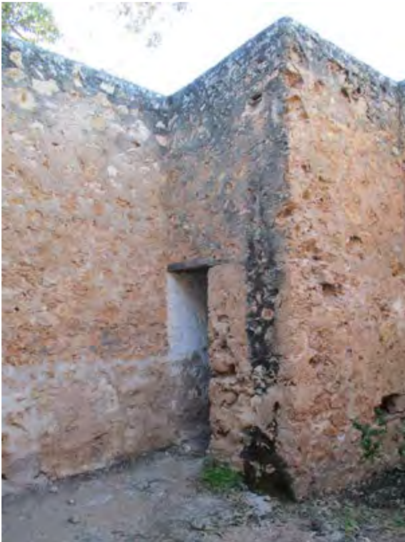
Figure 10: Section 95 prisoners were helping repair deteriorating stonewalls at the Greenough Hamlet heritage site.
