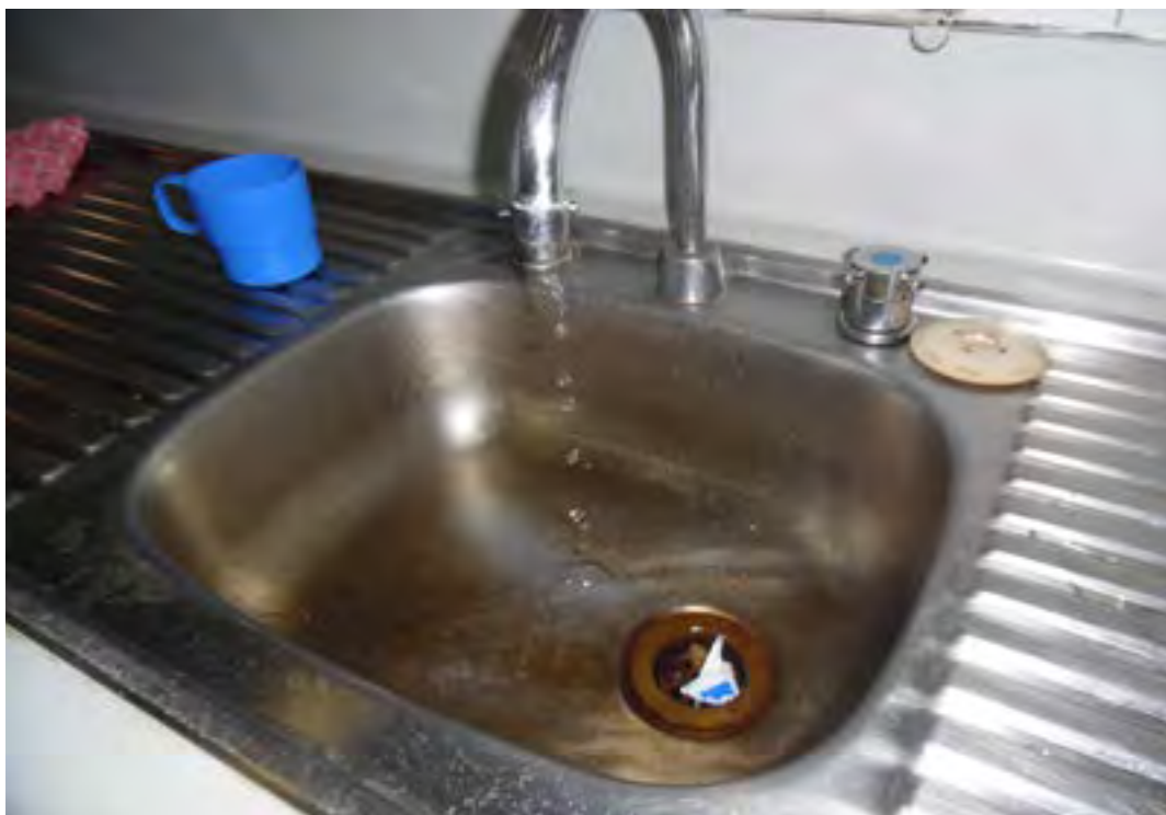
Figure 4: A leaky tap in Unit Four.
