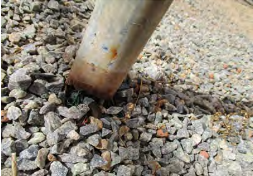
Figure 5: A rusting pole
