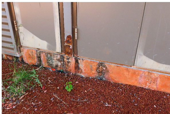
Photo 7: Water damage to concrete pad
