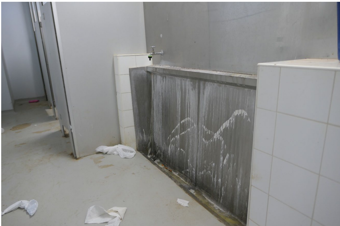
Photos 5 & 6: Unit bathrooms were unclean and untidy, with rubbish, visible staining, and calcification.
